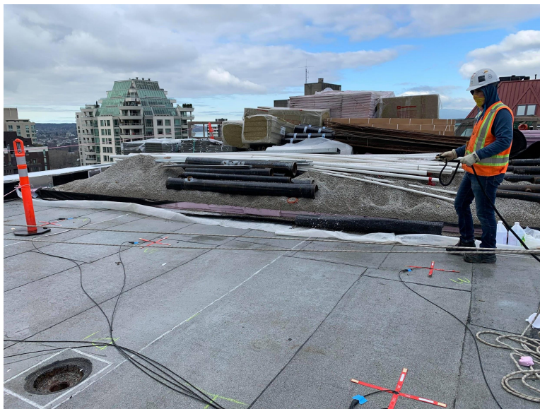
Above: FutureCast sensors sit on top of the waterproof membrane, and are covered by insulation and overburden.
