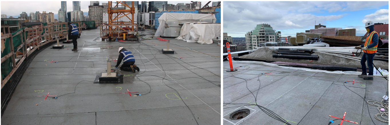
Above Left: FutureCast Digistar Sensors and EFT are applied directly onto the membrane. Above Right: The FutureCast sensors are attached to routed cable, and covered by roofing contractors.
