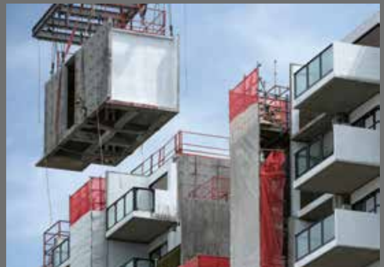
Avenue South Residence is the name of the world's tallest building to see the light of day thanks to modular construction. This high-rise is likewise being built in Singapore. By 2022, the twin towers will reach a height of 192 m and offer scope for more than 1,000 exclusive apartments. Special cranes are in place to lift the up to 30-ton modules into position correctly.
