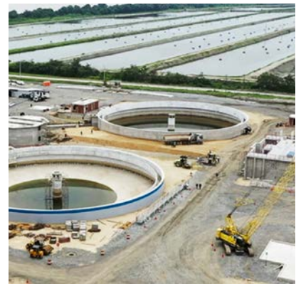
In Guayaquil, Ecuador, Sika is currently supplying products for a new wastewater treatment plant. One million apartments will be connected to the corresponding sewage system.
